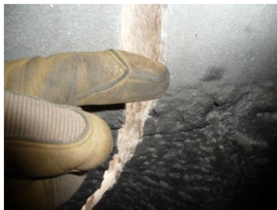
A crack in the Washington Monument's exterior wall caused by the August 23, 2011 earthquake.
